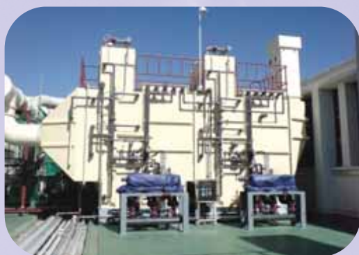
2 Stage IWS™ installed in LCD display plant in Korea to remove SiO 2 , HCl and HF for CVD exhaust gas
