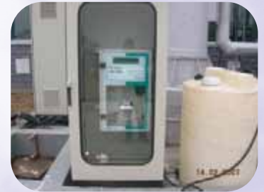
In-line titrator for controlling for chemical oxidant
